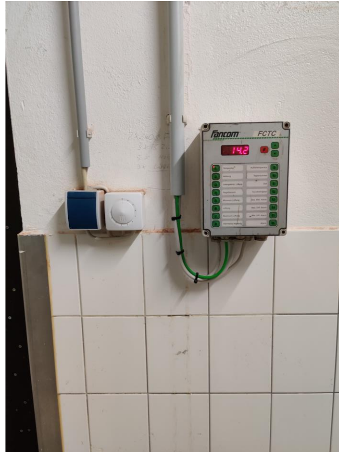
Controlling airflow, exhaust air, temperature
